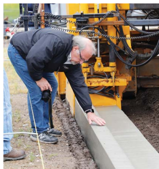
Dr. Michael Ayers inspects concrete curb and gutter with the MCE additive
